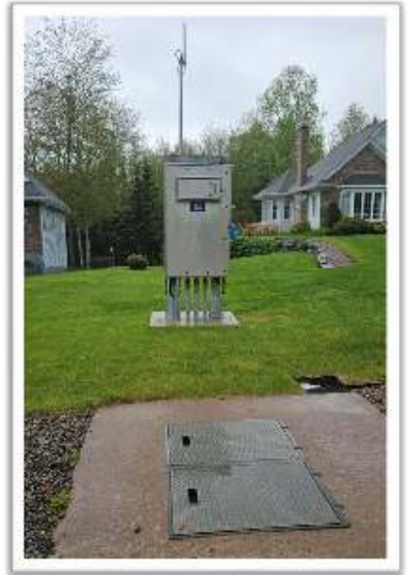
Example of Village Sanitary Sewer Pump Station
